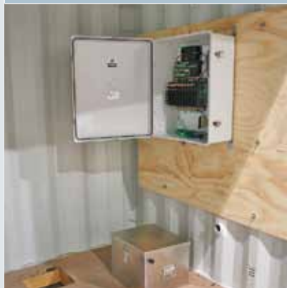
Above: Instrument/datalogger house designed inside a 6ft. container.
