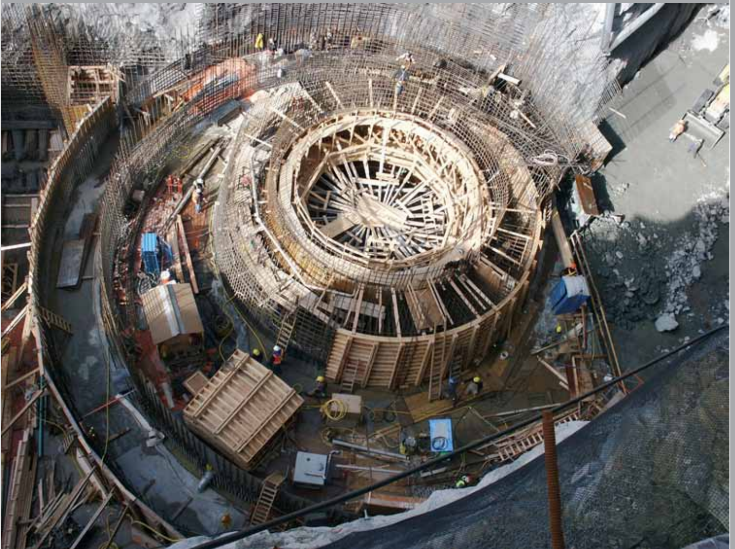
Thermistor installation for determining concrete curing temperature – Kaplan Turbine Scroll Case, Brilliant Dam – British Columbia, Canada
