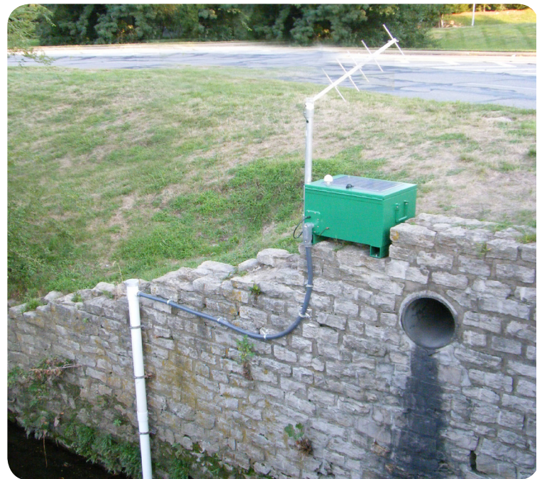
Portable aluminum chest monitoring system containing YSI Sonde and WaterLOG Data Logger. Kansas City, Kansas
