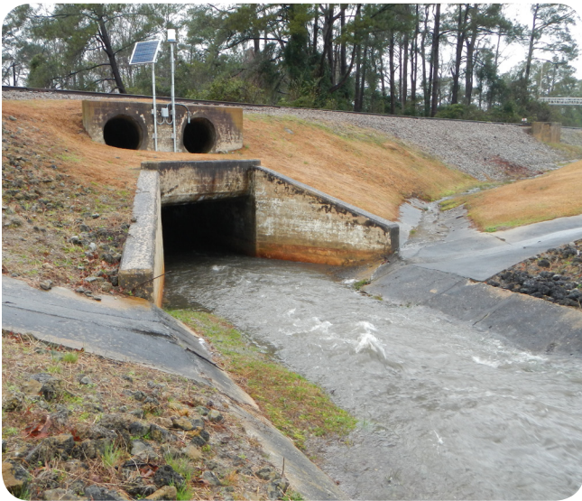
Stormwater monitoring site containing SonTek-IQ®, YSI Sonde, WaterLOG Rain Gauge, Portable water sampler, Customer Data Logger, and Solar Panel. Havelock, North Carolina
