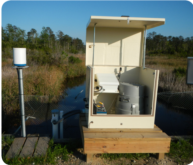
Portable fiberglass clamshell monitoring system containing SonTek-IQ®, YSI Sonde, WaterLOG Rain Gauge, Portable water sampler, Customer Data Logger, and Solar Panel. Havelock, North Carolina
