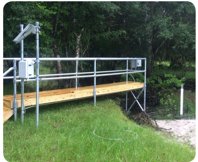
Stormwater monitoring site containing WaterLOG Radar, WaterLOG Data Logger, and Solar Panel. Greenville, South Carolina
