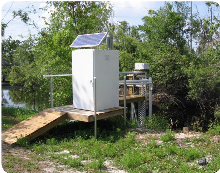
Stormwater monitoring site containing SonTek-SL, WaterLOG Shaft Encoder, YSI level sensor, YSI Sonde, Portable water sampler, WaterLOG Rain Gauge, YSI Data Logger, and Solar Panel. Kissimmee, Florida
